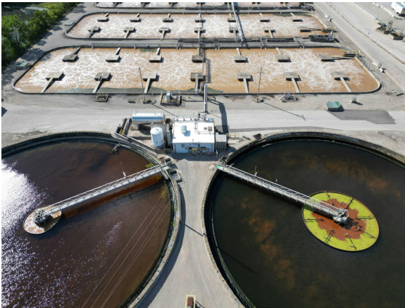
F68. Stormwater Infrastructure (Pexels, 2025)
